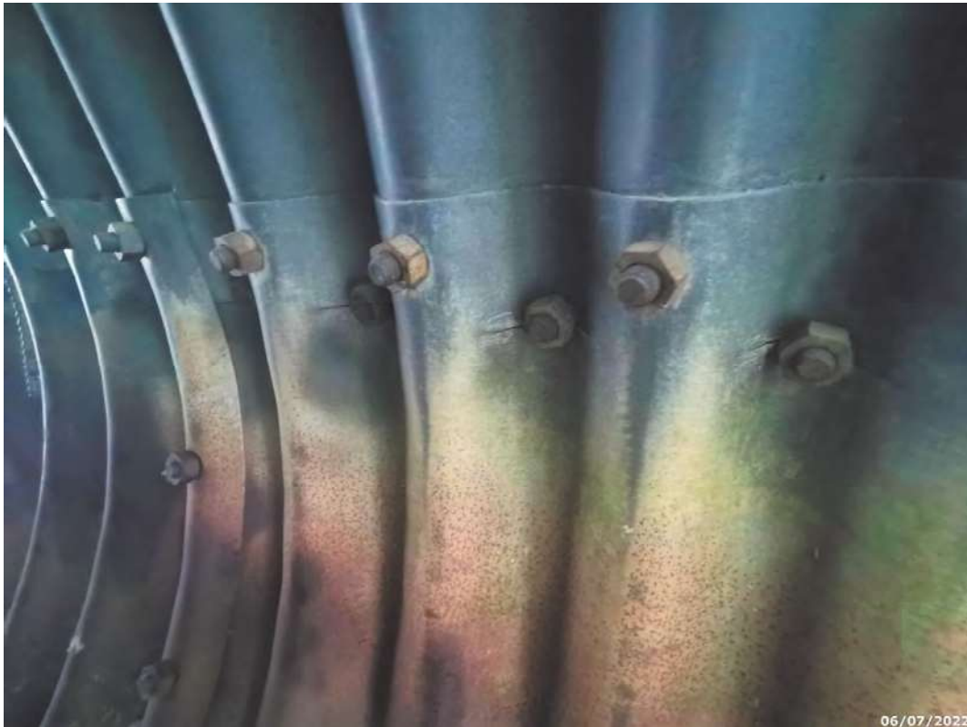
Cracking at Bolt Line Along West Wall
