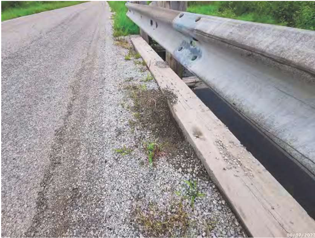
Curb/railing system with excess gravel buildup on bridge deck
