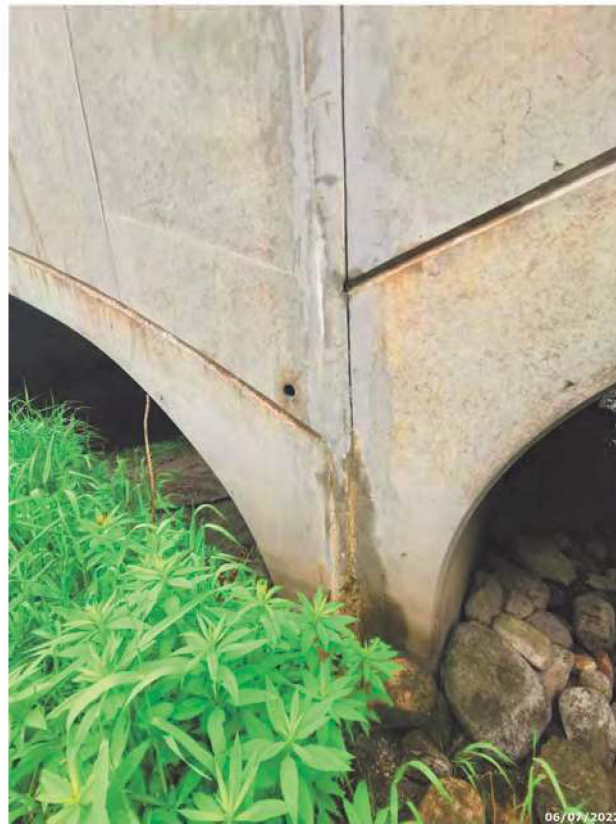
Moisture and wetting of center joint
