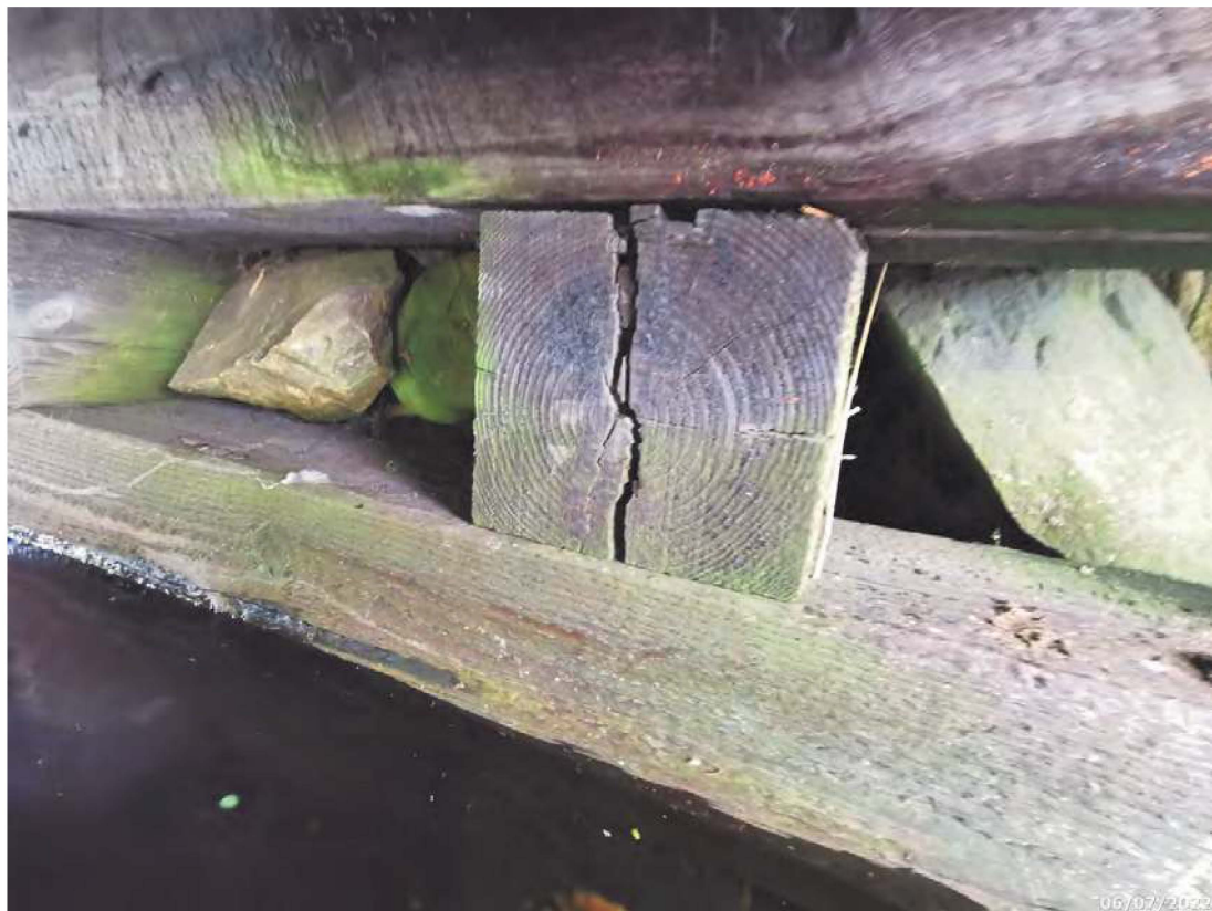
Wide split in second timber from north in cribbing
