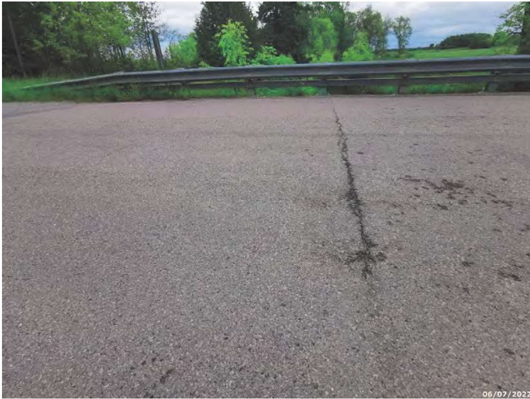
Medium to wide transverse crack in north approach
