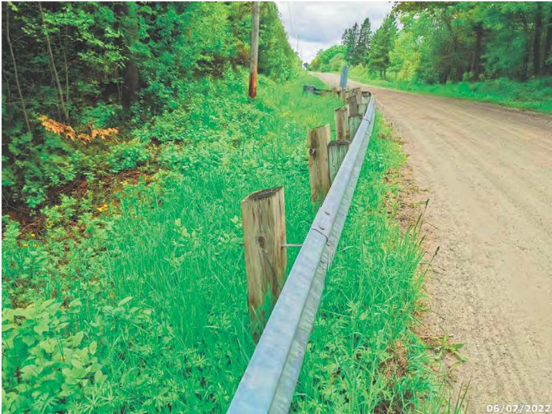
Rotated approach guiderail and missing spacer block, southwest approach
