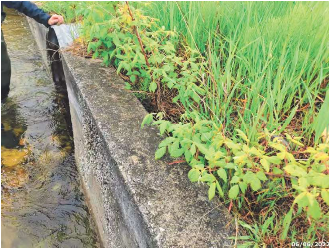
Light pop outs and erosion behind concrete headwall. (NW quadrant of bridge)
