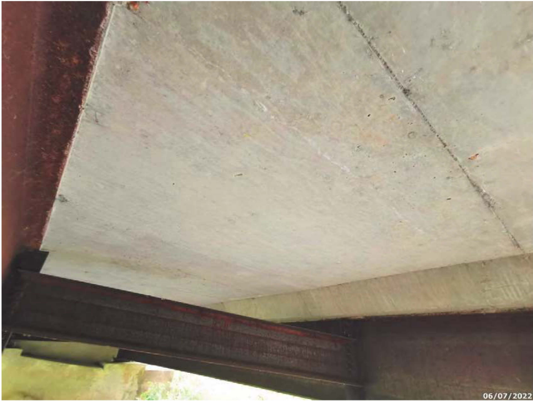
Localized crack with efflorescence
