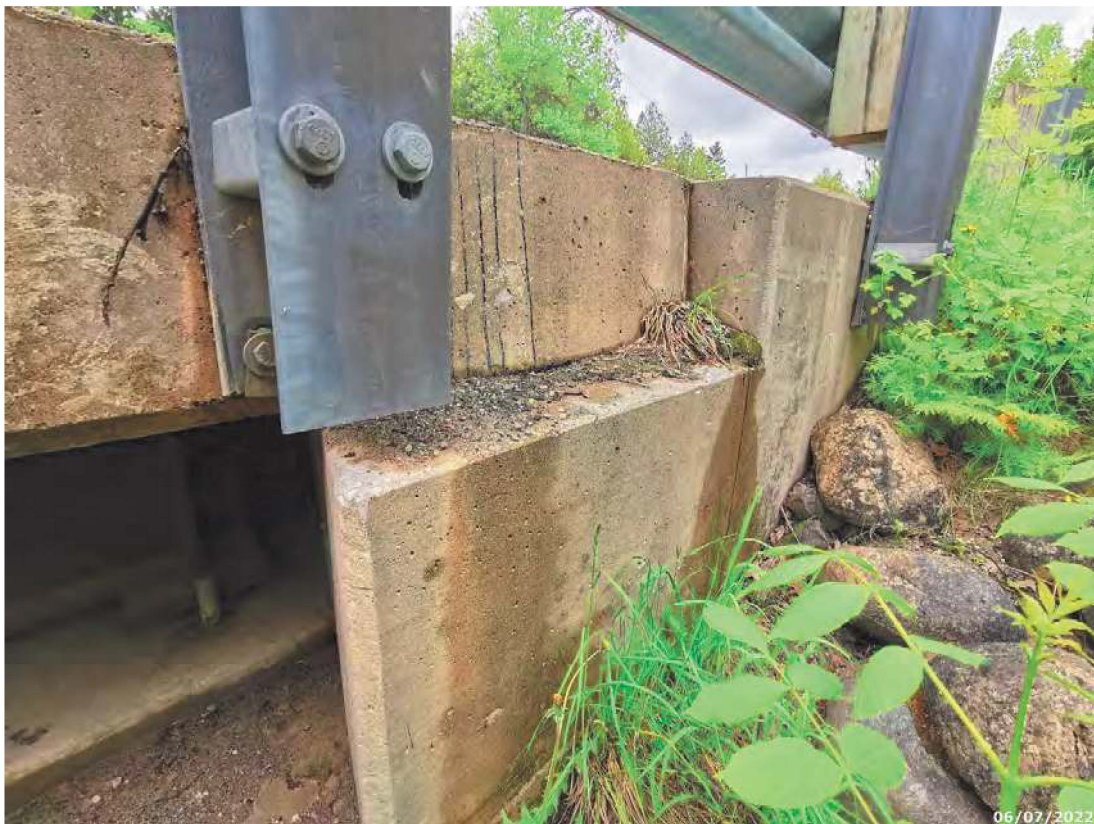
Debris buildup in bearing seat
