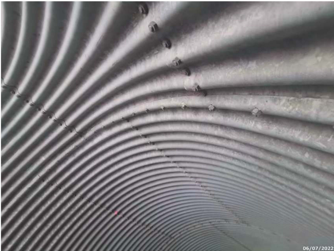
Center line joint, no full contact of nuts
