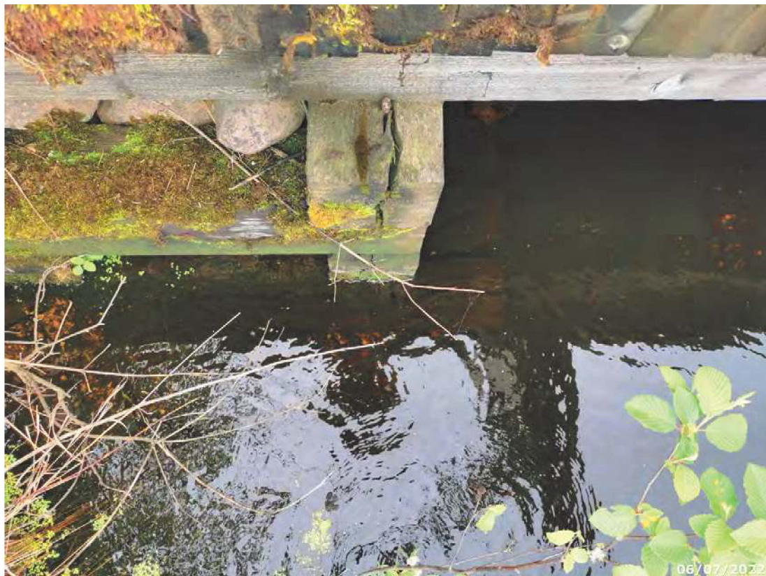
Northeast abutment cribbing with moderate decay, lichen growth and wide split through dowel
