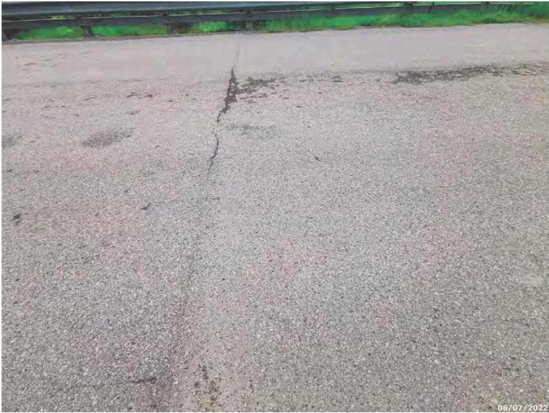
Light to medium transverse crack and settlement of south approach wearing surface
