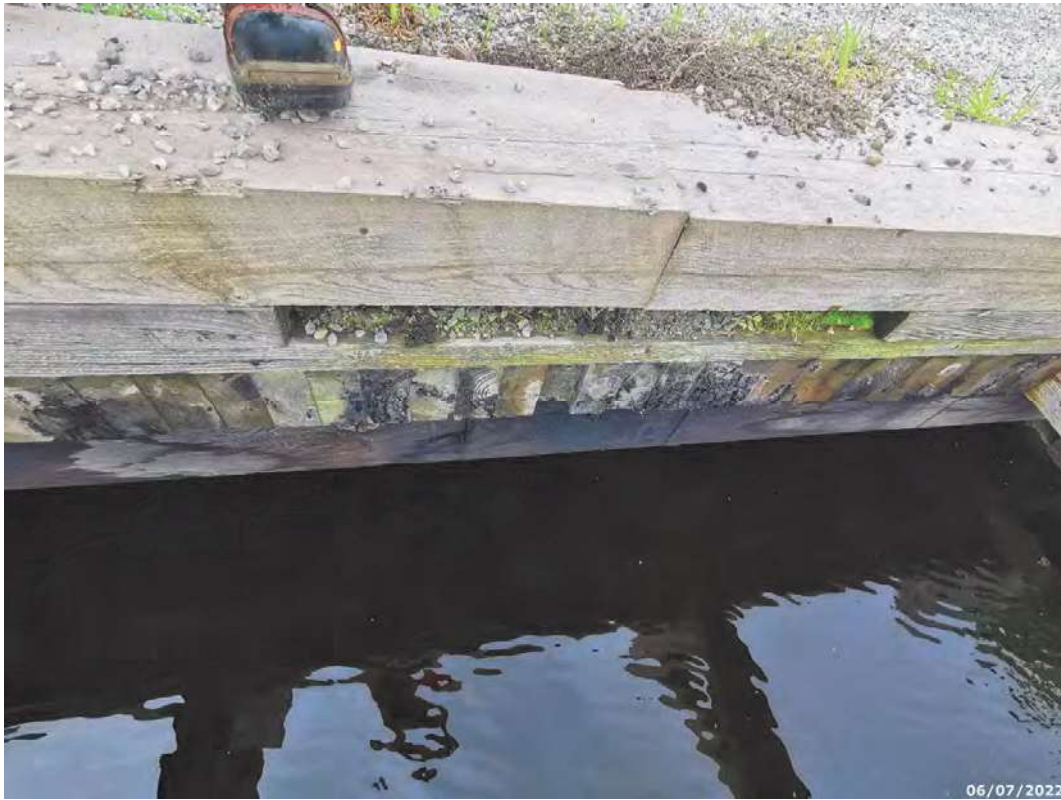
Plugged scupper drain in curb
