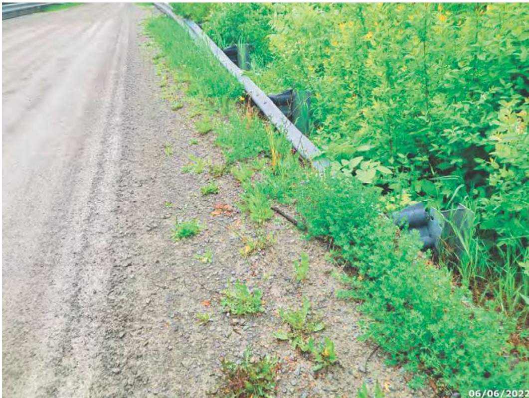
Northeast approach guiderail, broken spacer block, vegetation encroaching
