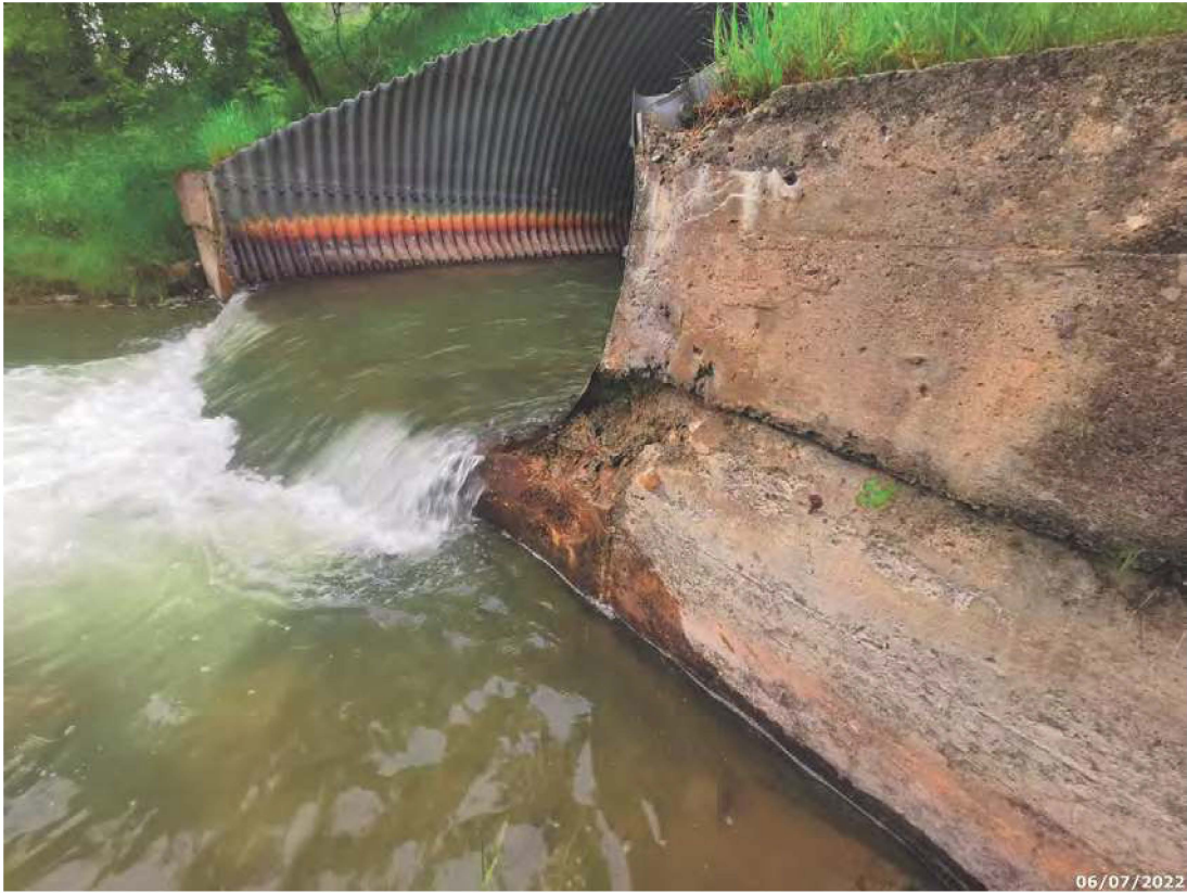
Moderate spall on southeast outlet cutoff wall
