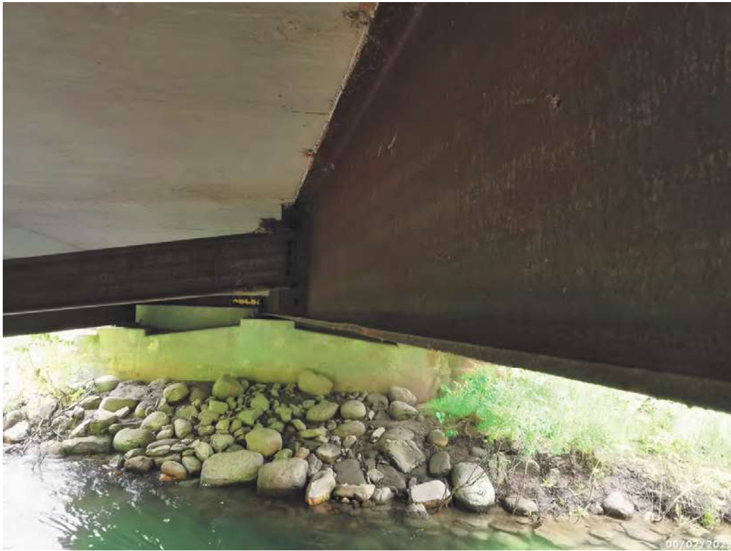
Channel brace, local deformation in girder bottom flange
