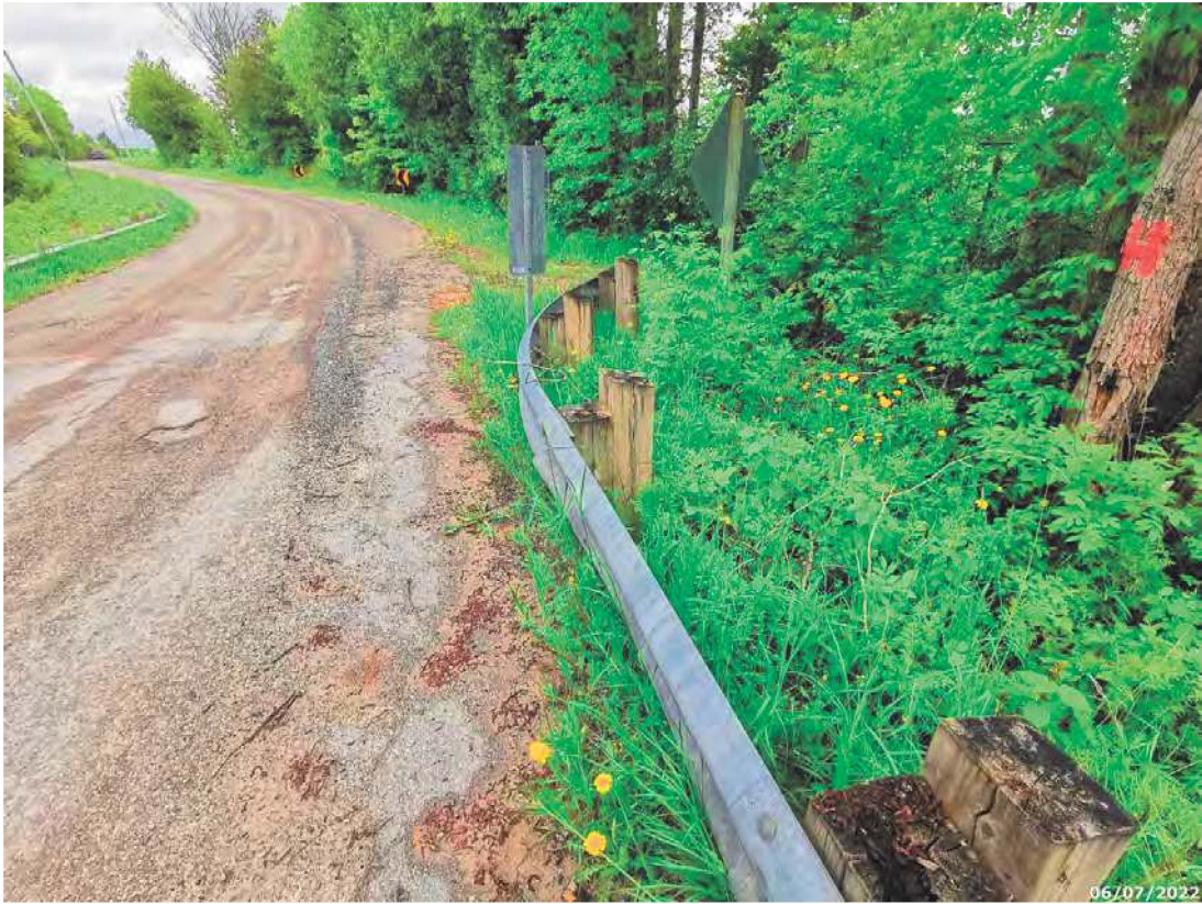
Severe end decay of spacer block
