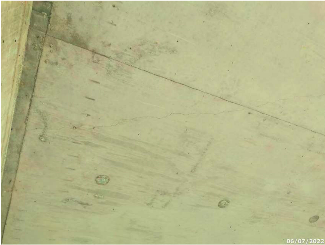
Medium crack in soffit in southeast quadrant
