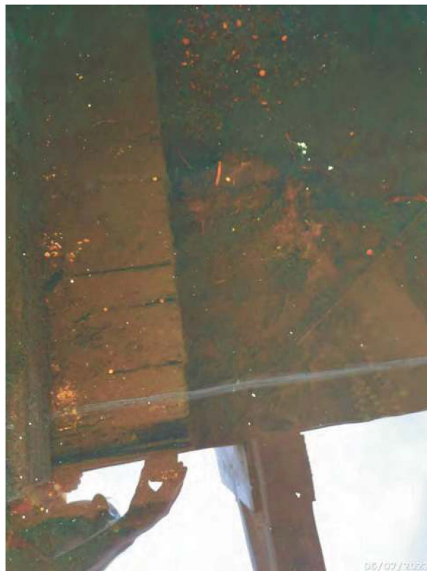
Typical footing undermining
