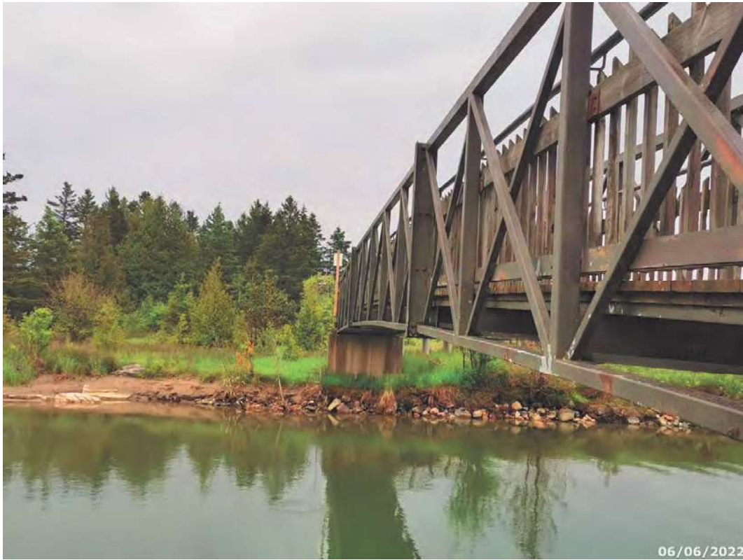
Moderate deflection of bottom chord at midspan
