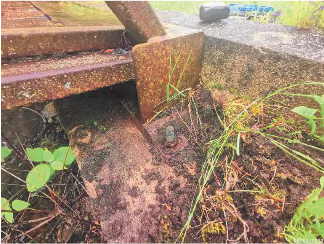
Severe debris buildup, south bearing
