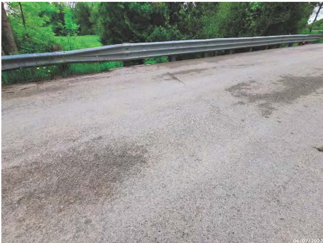
Settlement of east approach
