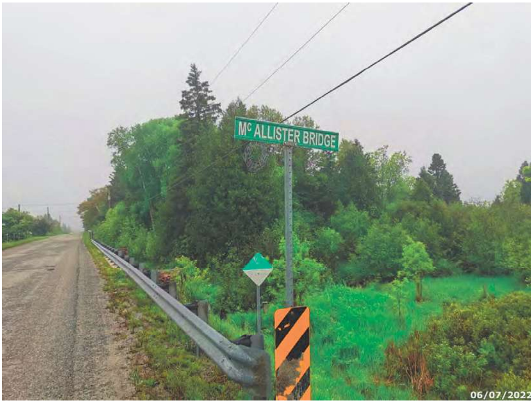
Bridge sign and dirty hazard marker
