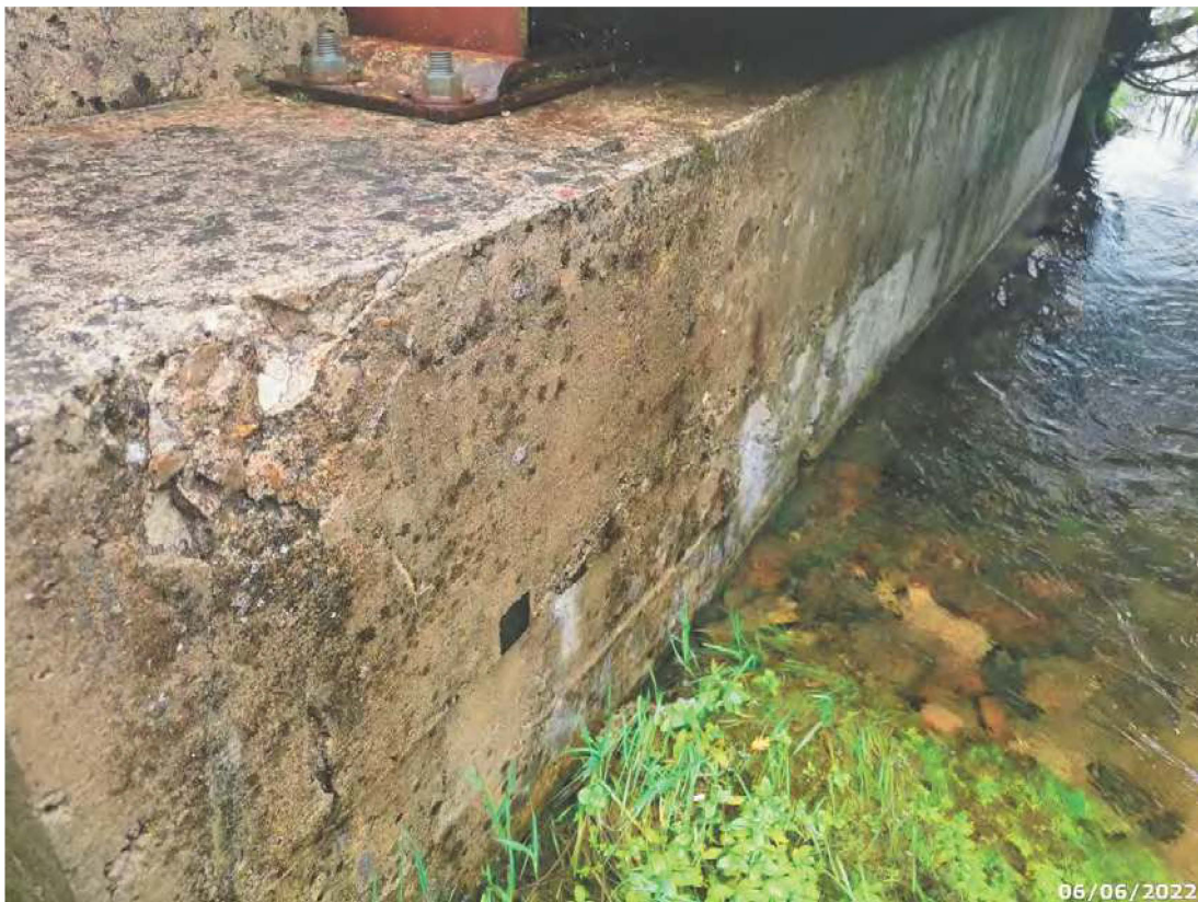
North abutment general arrangement, light spall and undermining at south edge
