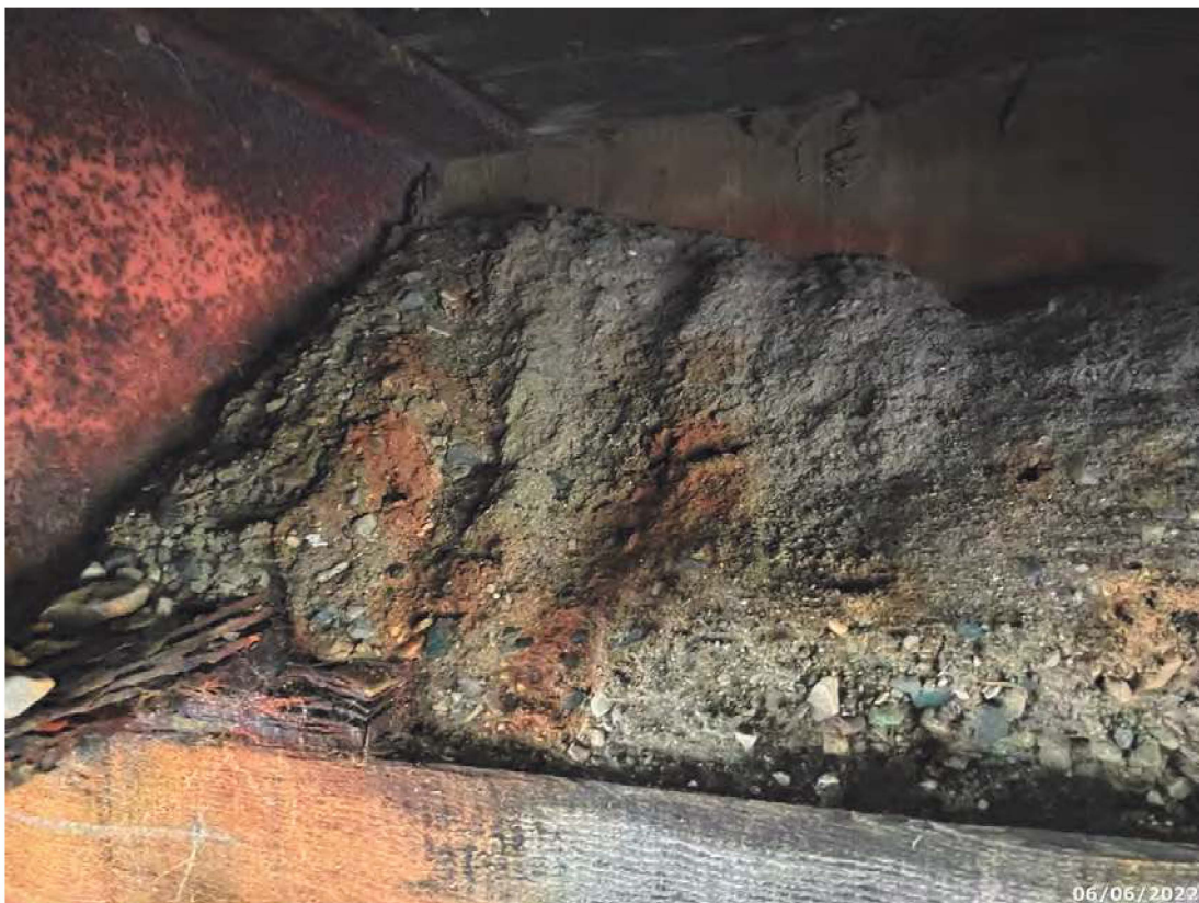
Severe debris build up at bearings
