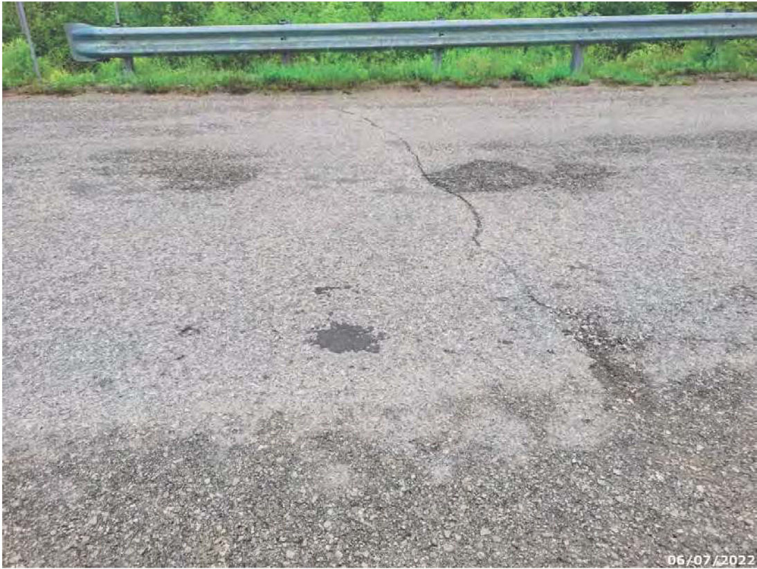
Medium transverse crack in north approach
