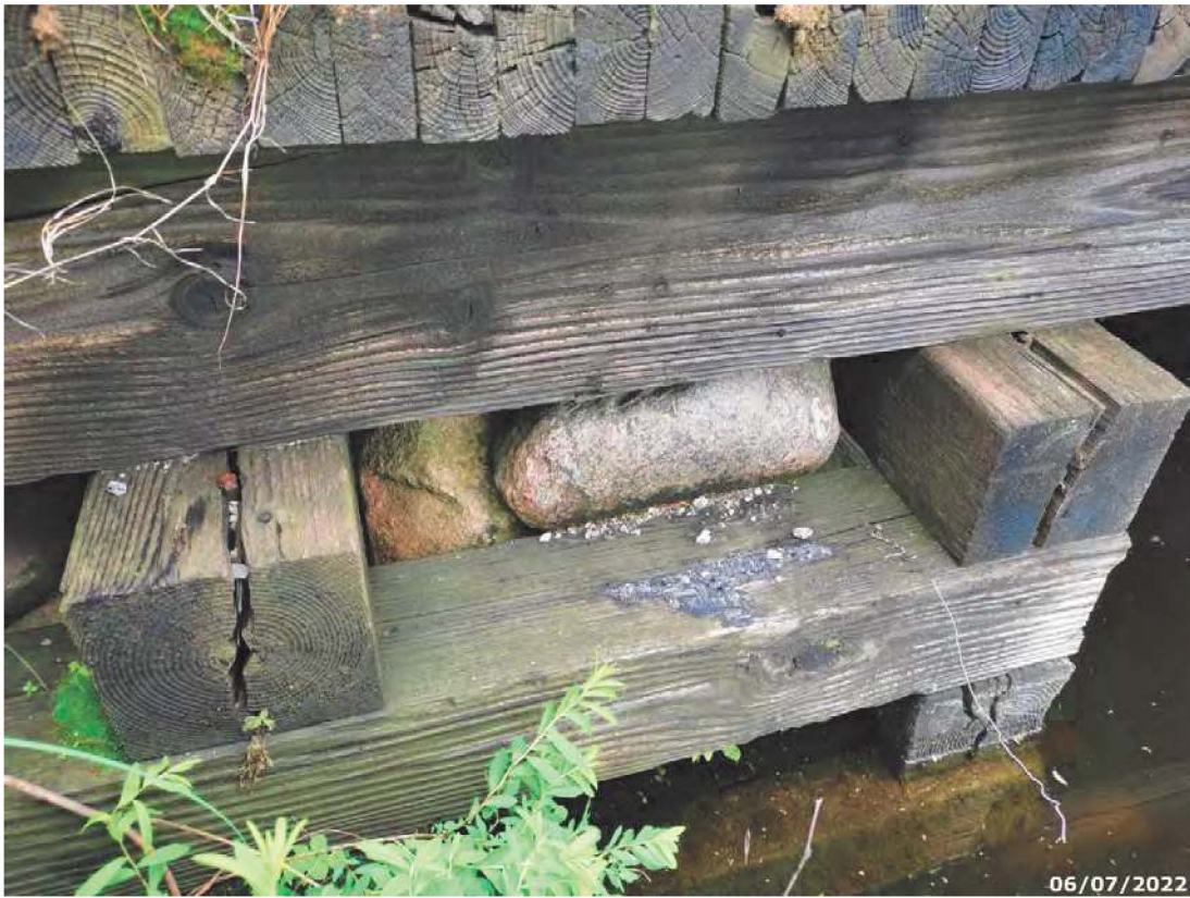
Wide splits in cribbing members
