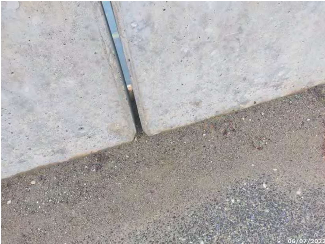
Sand buildup at south barrier
