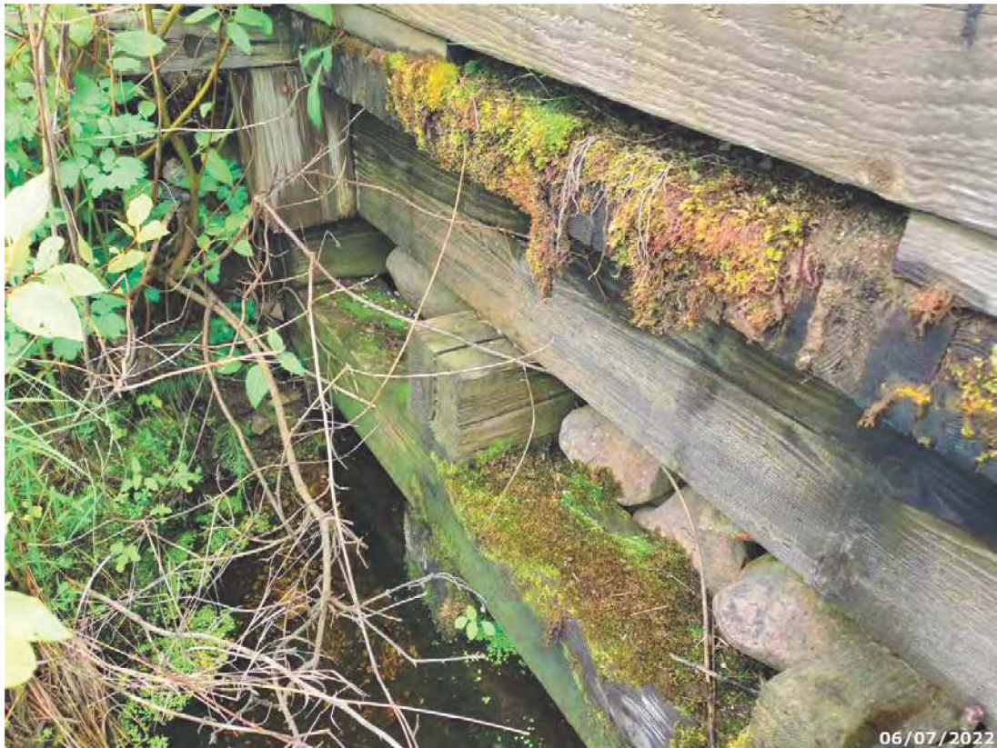
Typical edge of deck with algae and lichen growth
