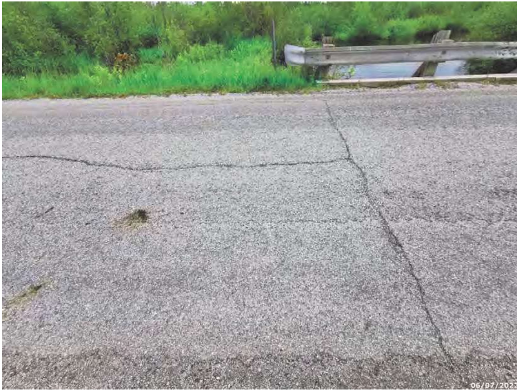
Wide transverse and longitudinal cracks at east approach
