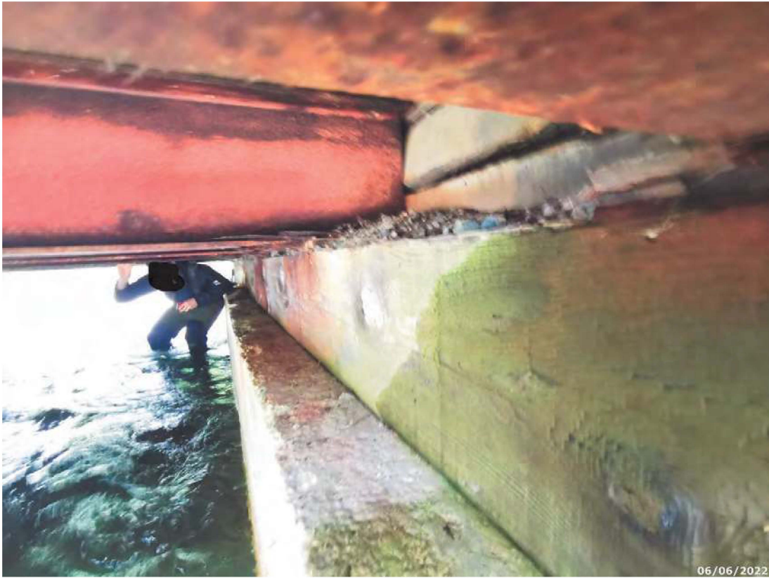
Severe corrosion of bottom flange and web at the west abutment.
