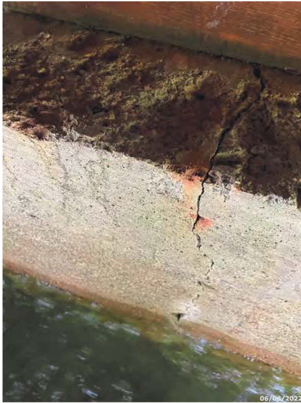
Wide crack in west abutment
