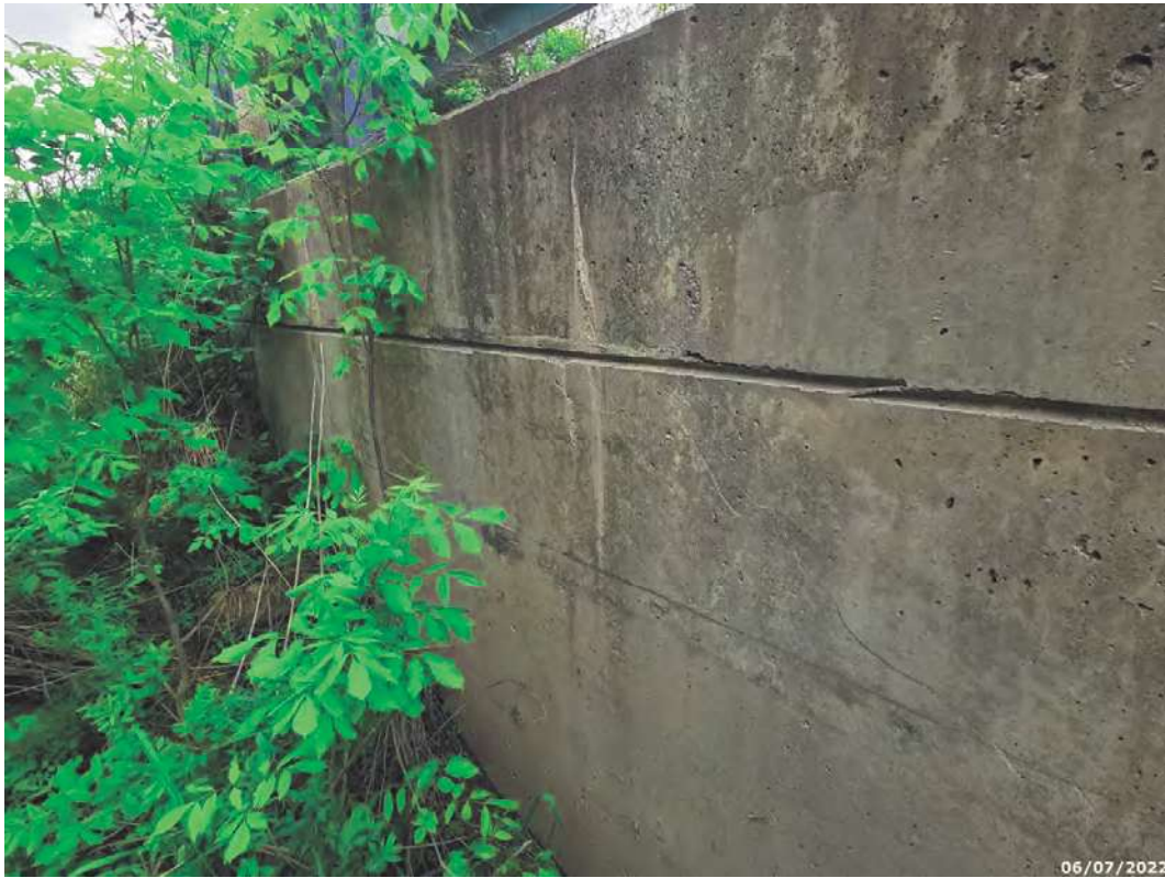
Localized stained medium crack at northwest wingwall
