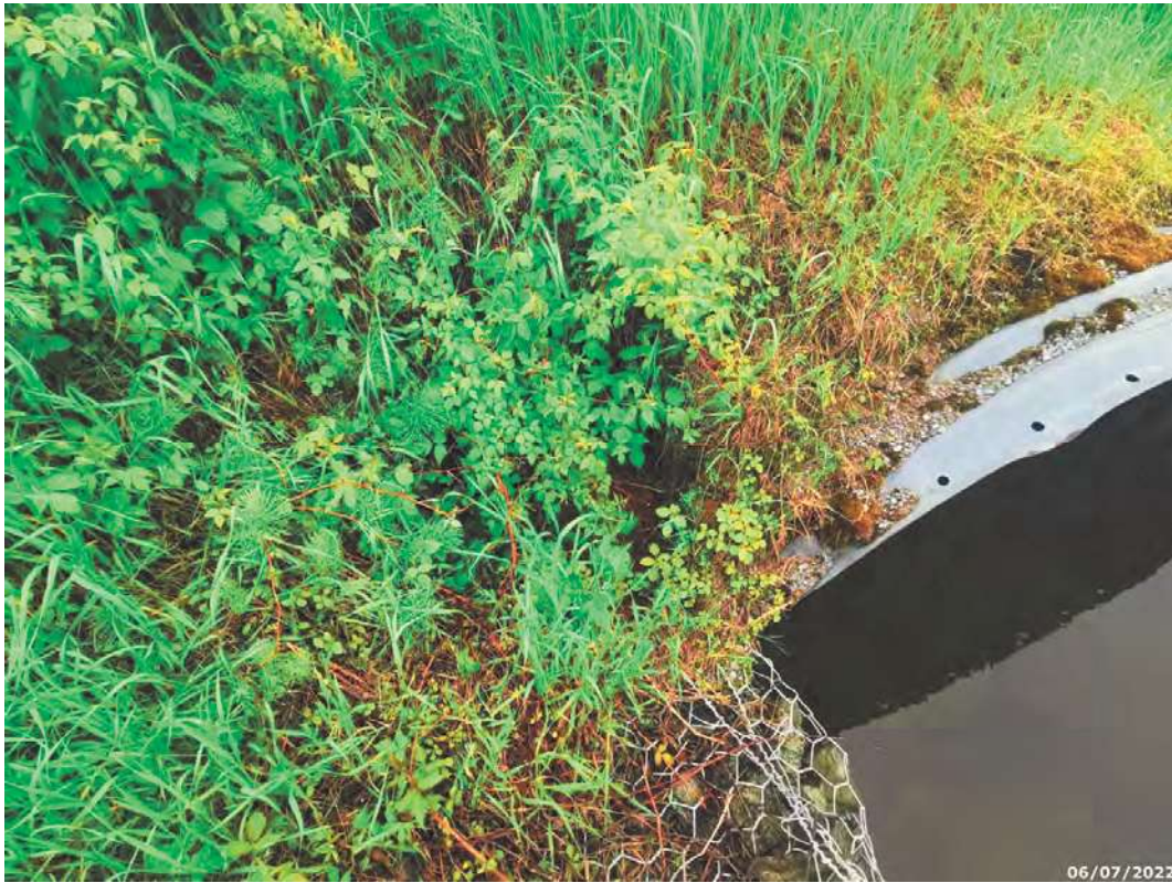
Erosion channel behind failed gabion basket
