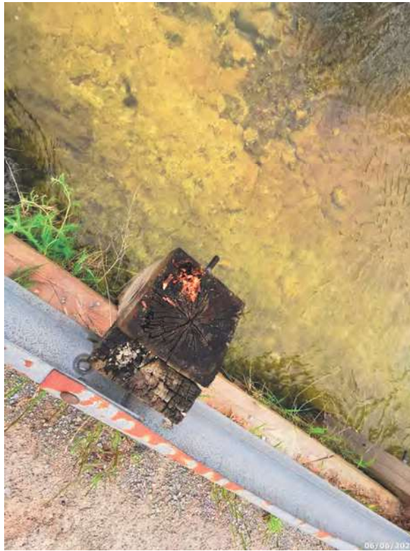
Typical decay of barrier posts
