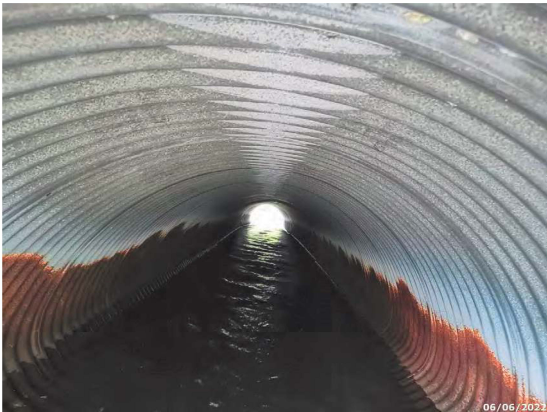
Sag in overflow pipe in obvert and dent at centerline
