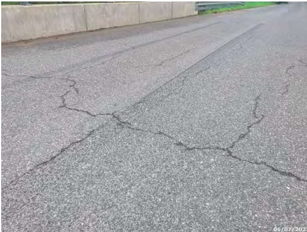
Light to medium map cracking in bridge deck wearing surface
