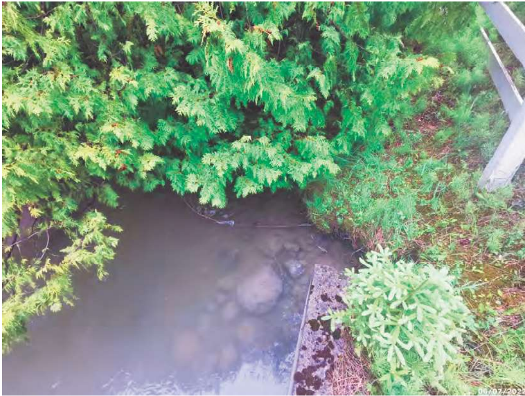
Moderate to severe scour and erosion at northeast quadrant
