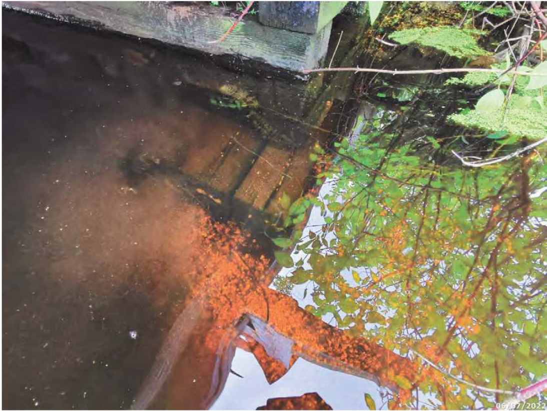
Typical footing with undermining
