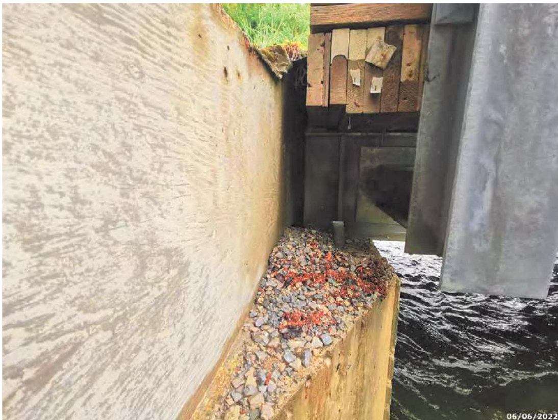
North abutment typical bearing, severe debris buildup
