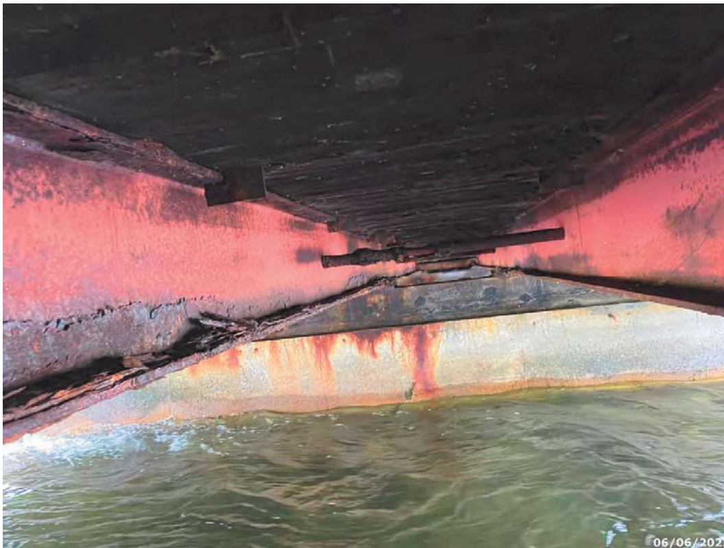
Severe corrosion in bottom flange, predominantly on centerline girder only
