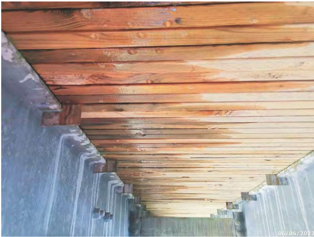
Actively wet exterior deck boards
