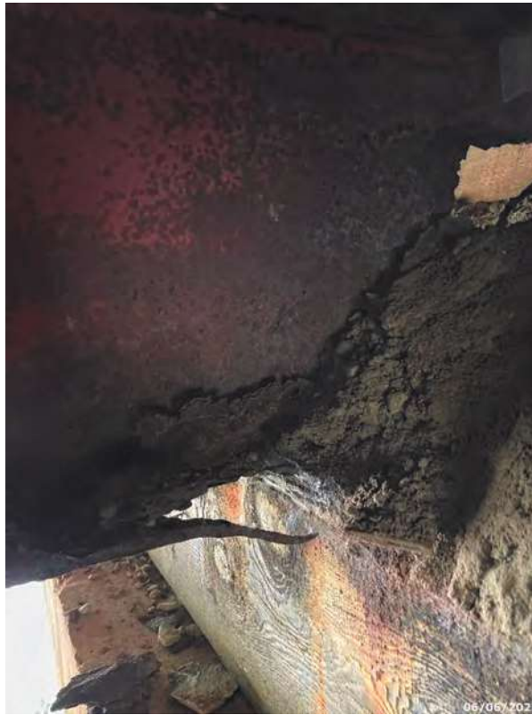
Severe Section Loss at Bearing
