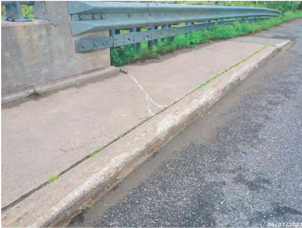
Sealed wide crack in approach sidewalk
