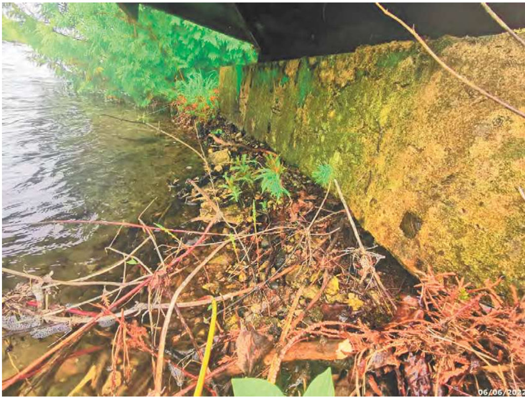
Moderate to severe undermining at south abutment
