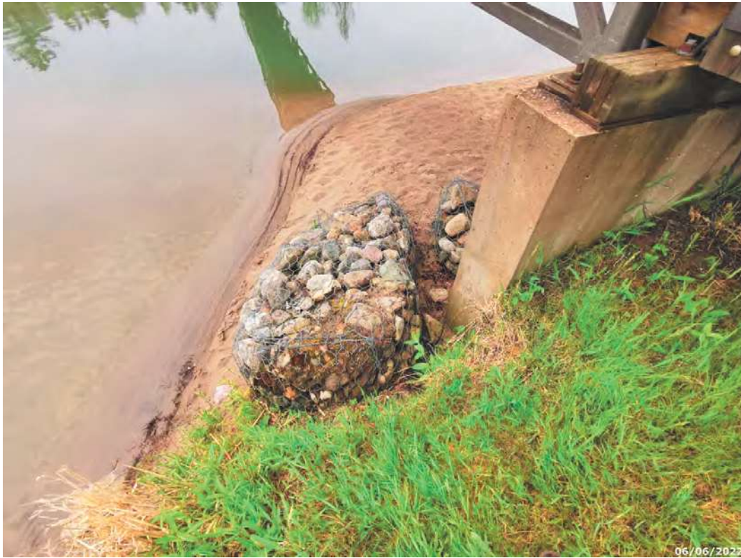
Failed and rotated gabien basket
