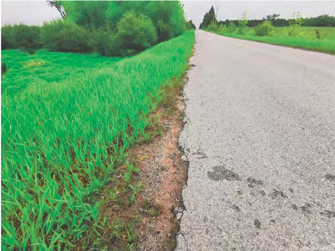
Potholes and broken shoulder edge of surface treatment
