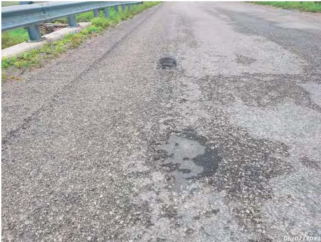
Localized potholes and patching
