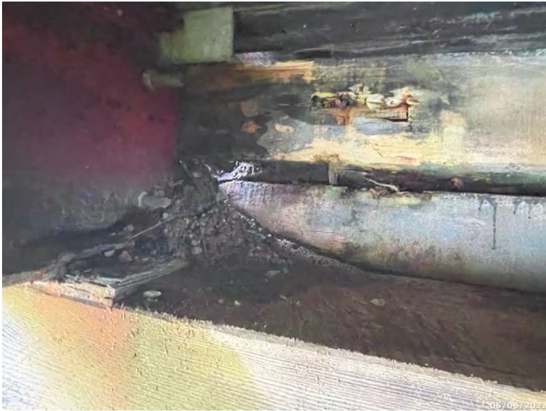
Severe Decay in Ballast Wall - Typical
