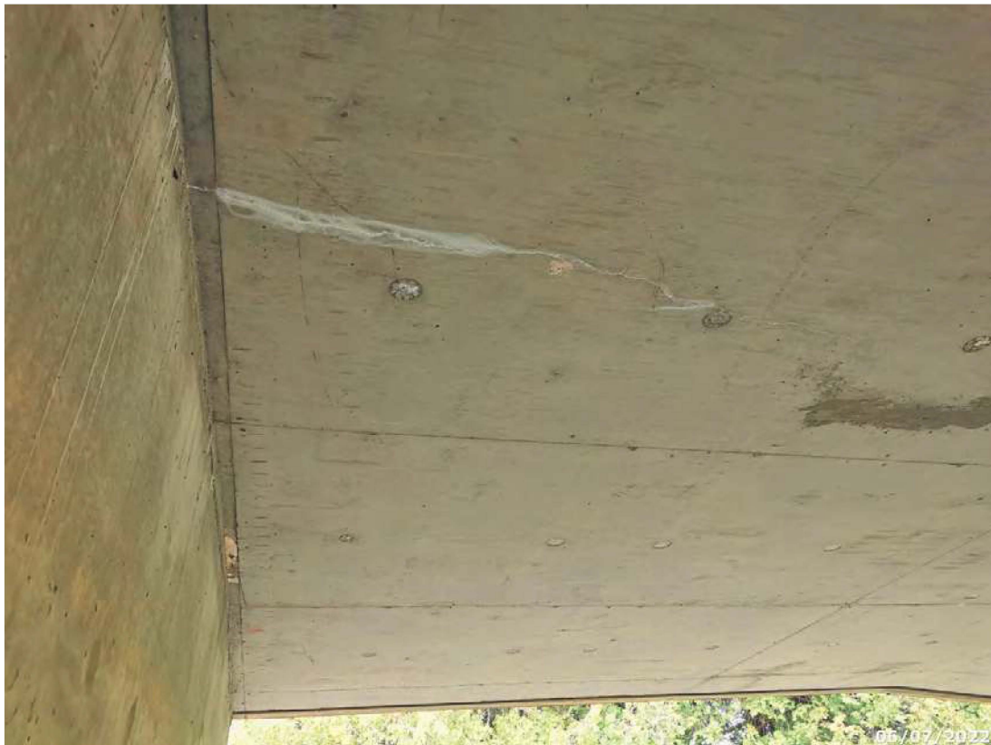
Medium to wide stained crack in soffit
