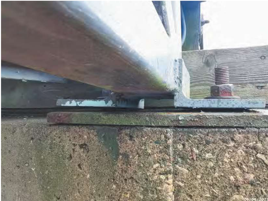
Minimal contact at northwest bearing
