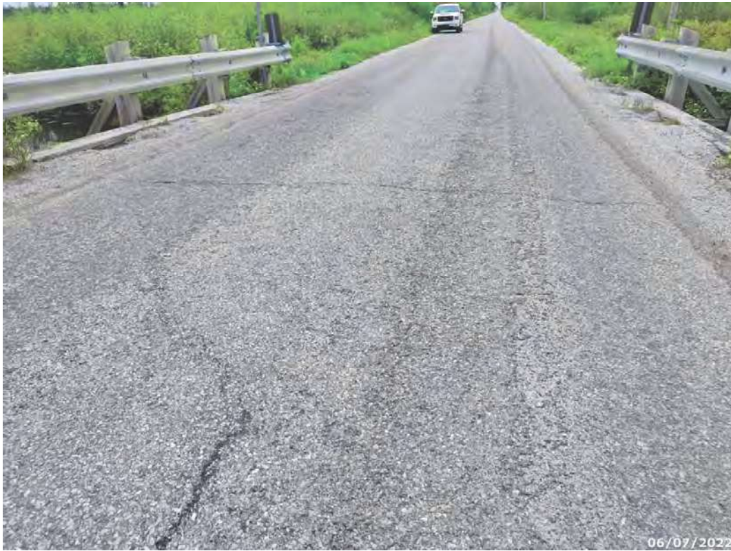
East approach with medium center line crack and wide transverse crack
