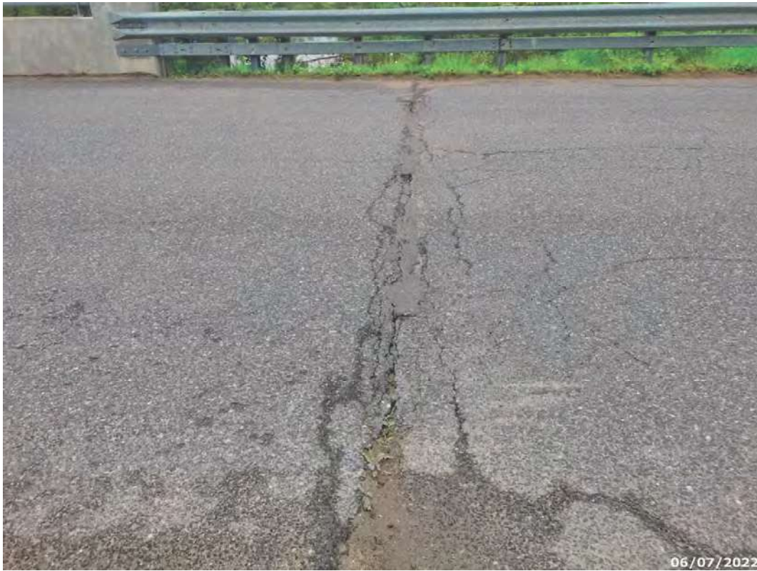
Wide transverse cracking and potholes at end of approach
