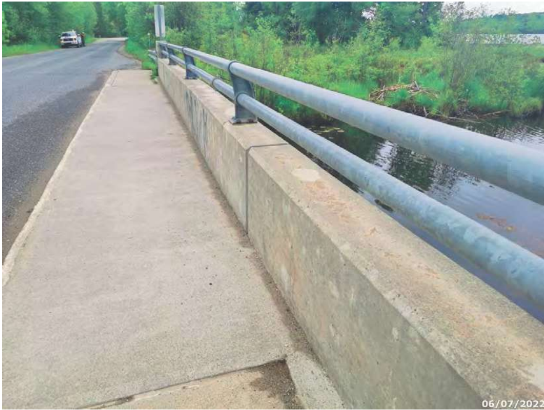
Typical barrier and handrail
