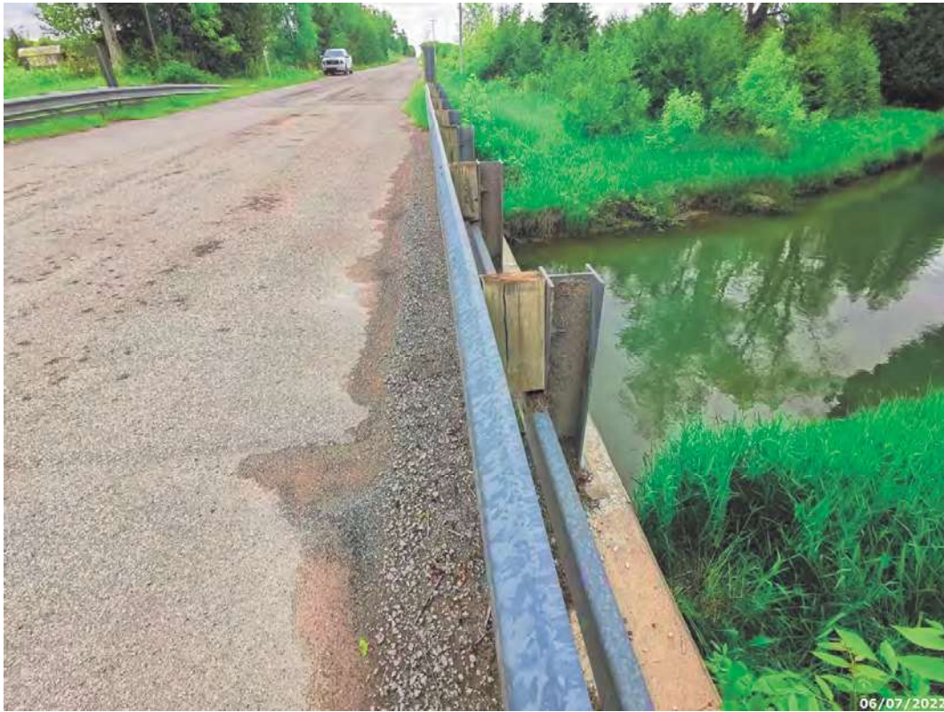
Typical barrier system, excess debris buildup
