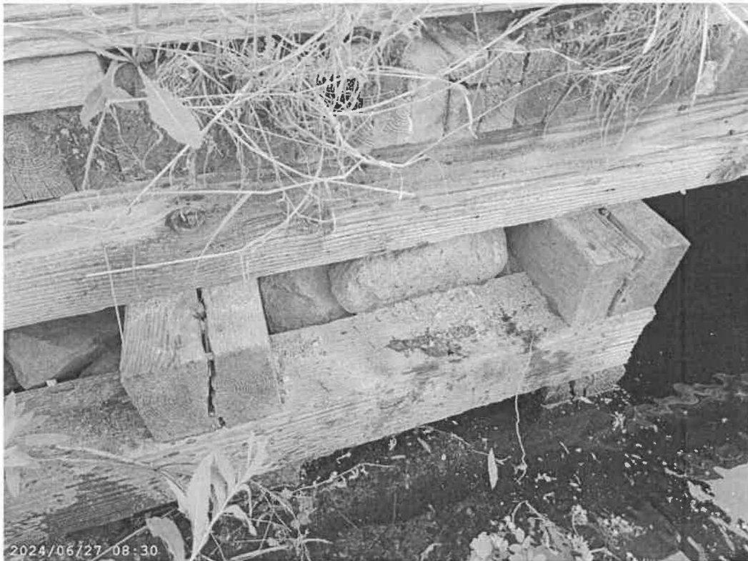
Wide splits in West crib at drift pins
