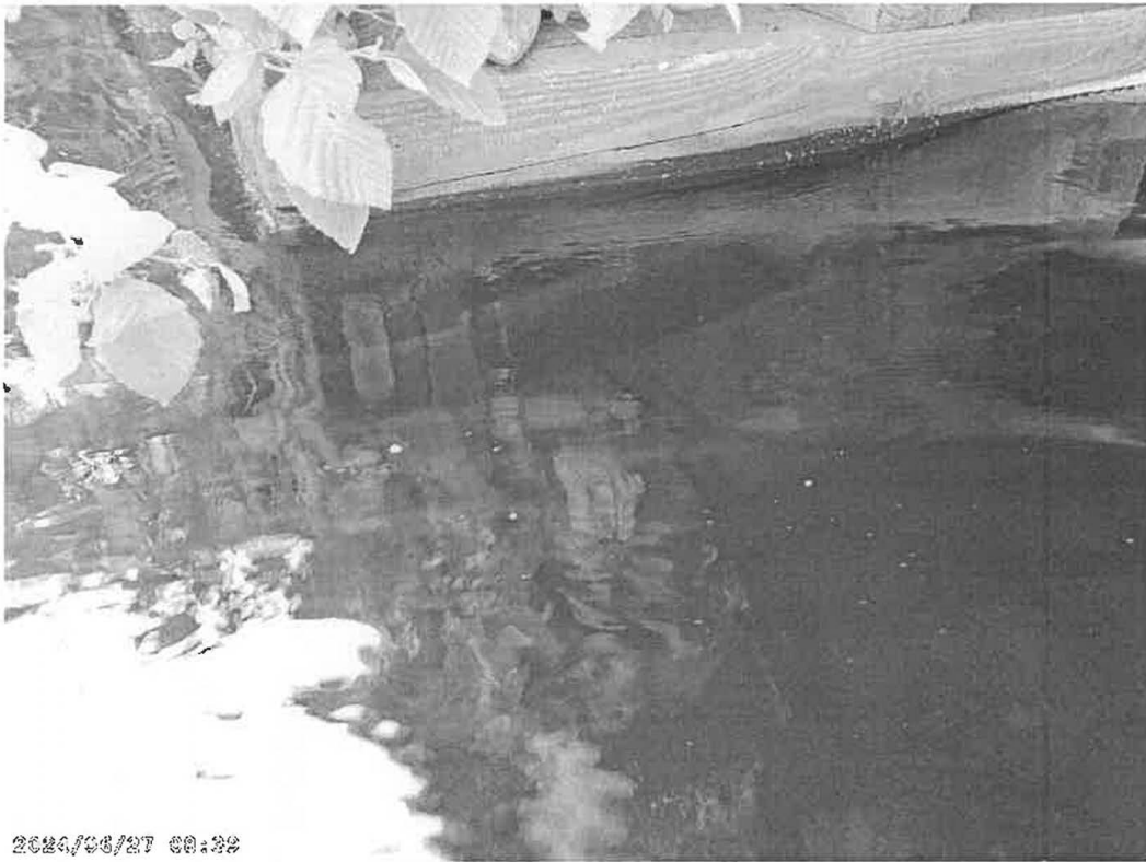
Exposed toe of cribbing bottom course bearing pad
