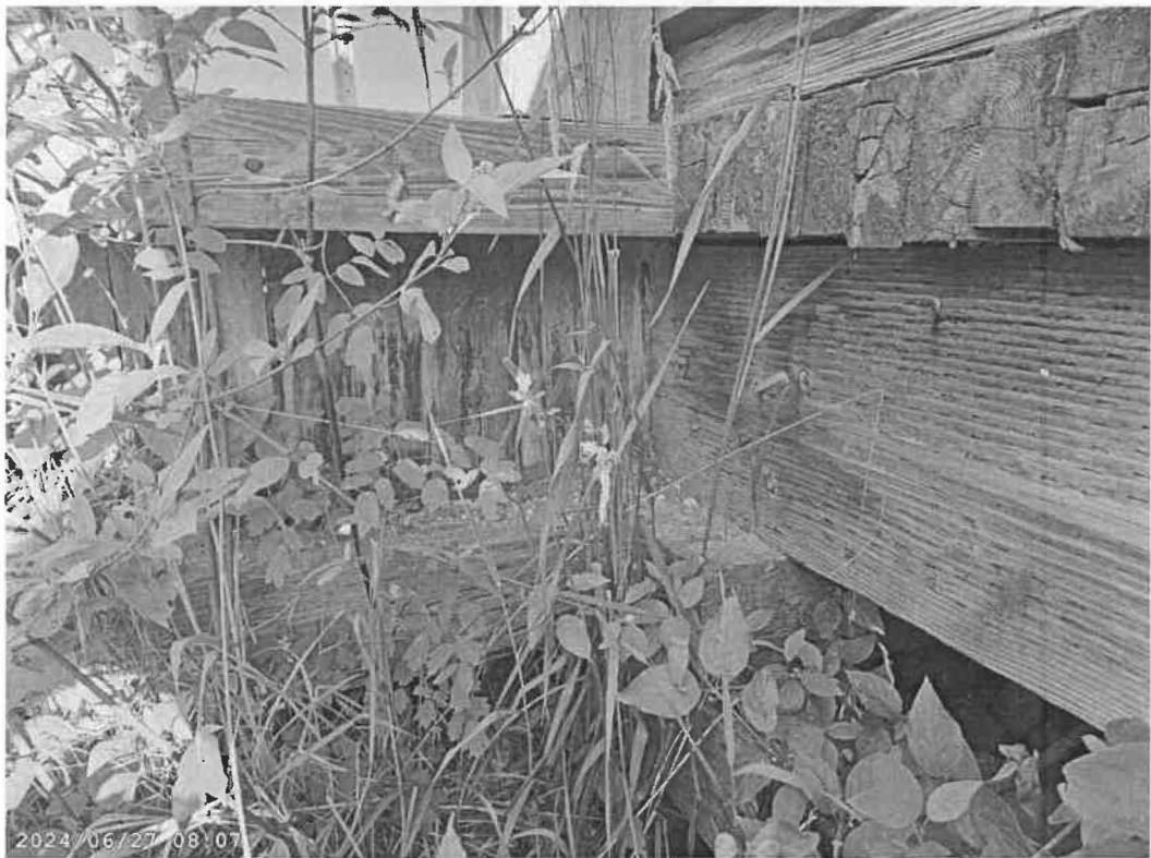
Light debris at bearing
