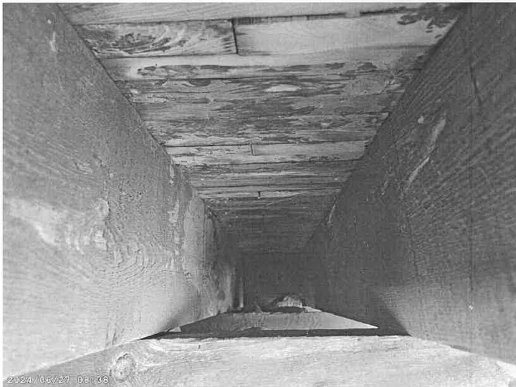
Water staining at edge of deck soffit
