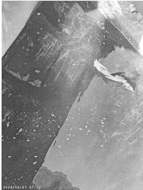
Exposed projection at front of crib with undermining
