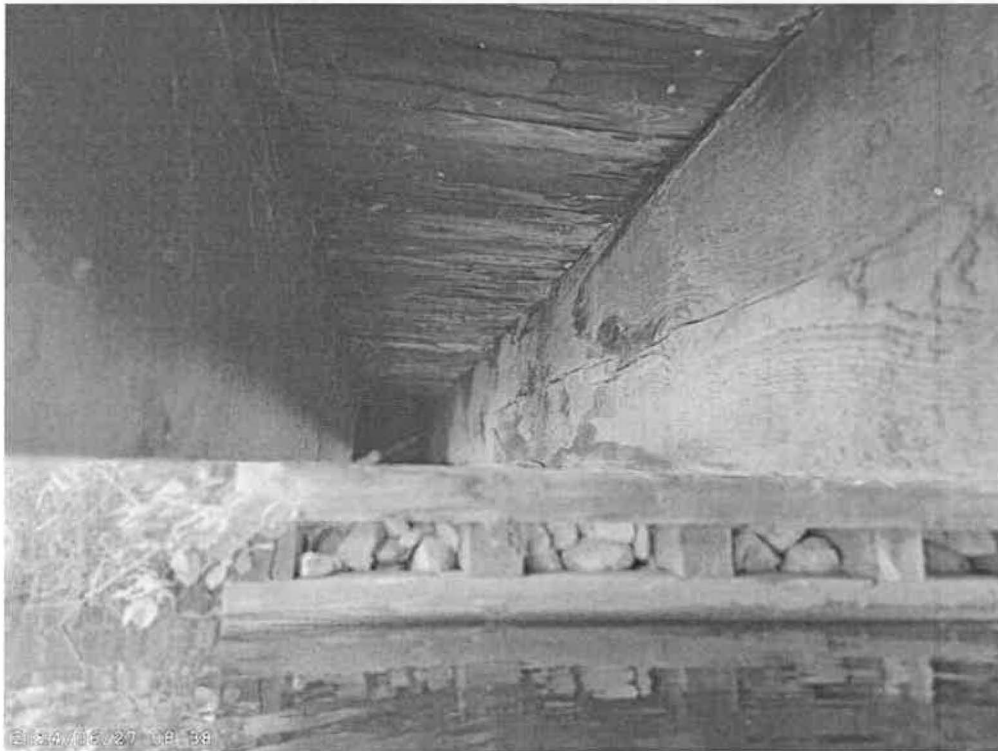
Exterior soffit and water staining on edge of stringer
