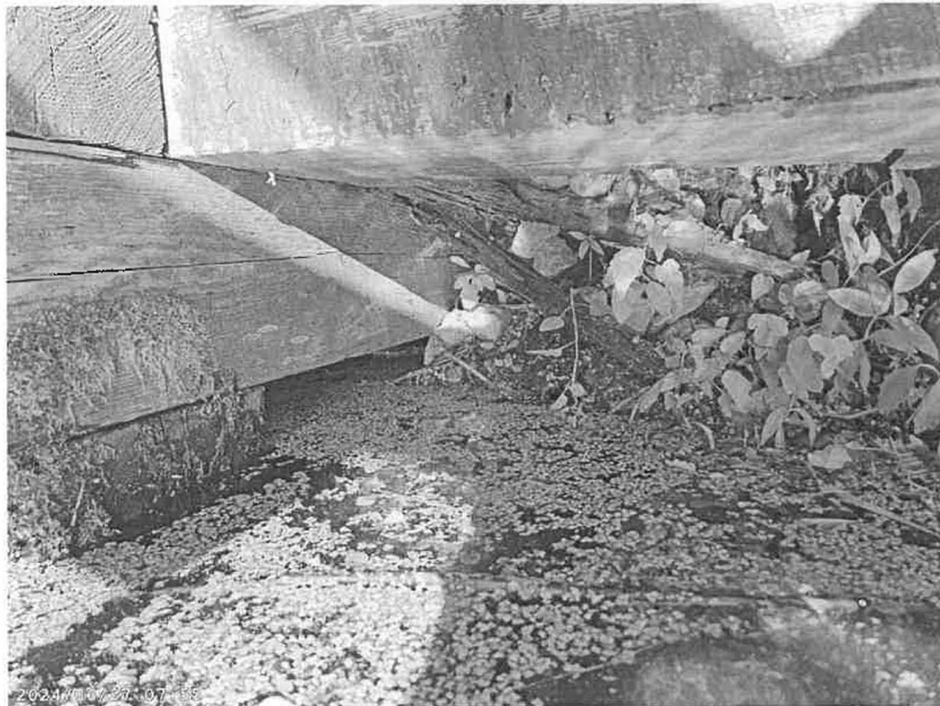
Failed ballast wall
