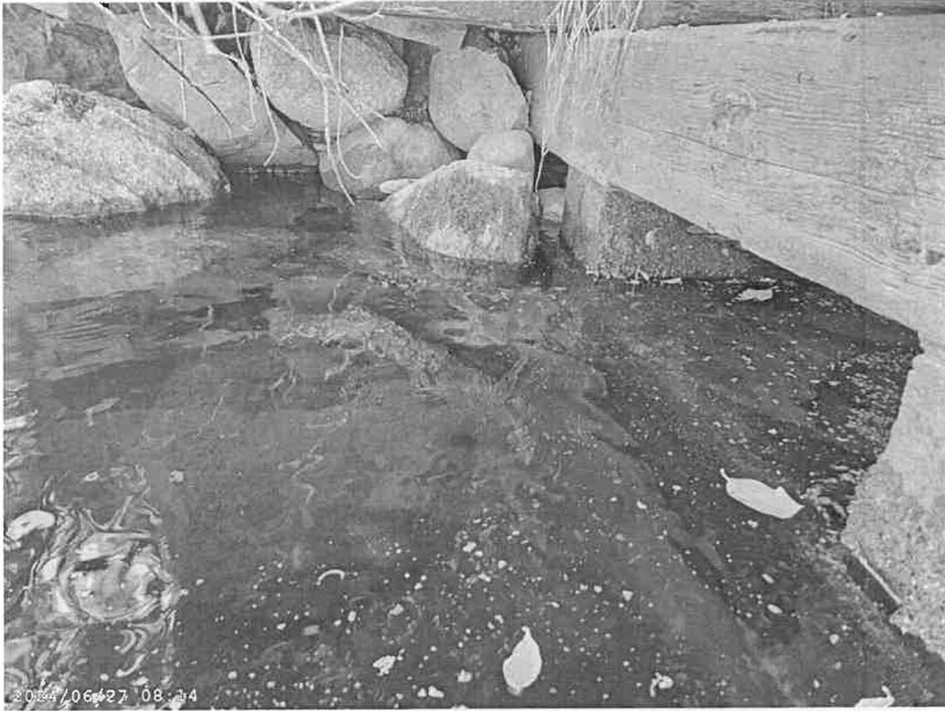
Loss of rock upstream (end of east abutment)
