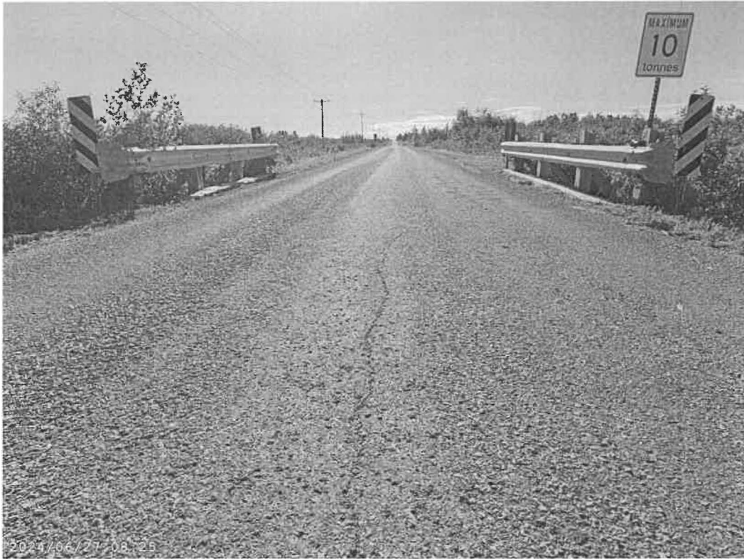
Medium longitudinal crack and typical wearing surface
