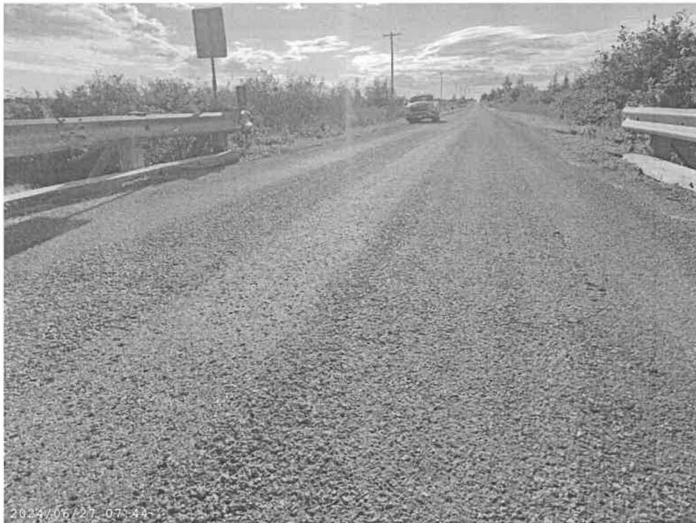
Wearing surface with light raveling, wear and rutting in wheel paths
