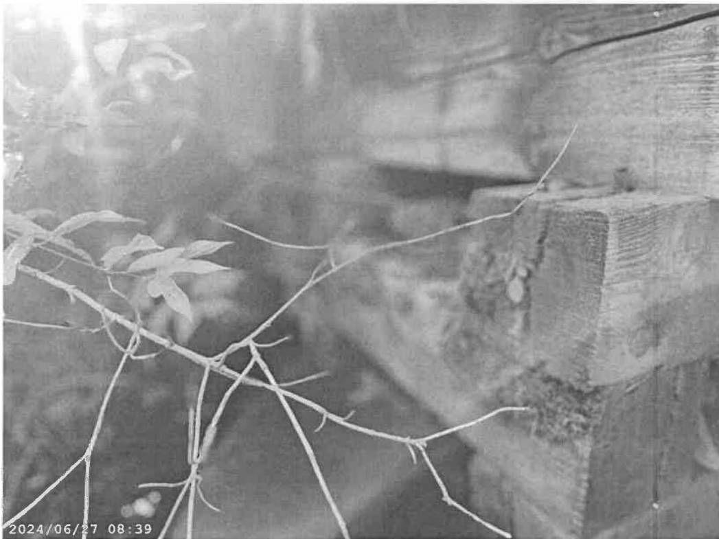
Algae growth on edge of East abutment cribbing
