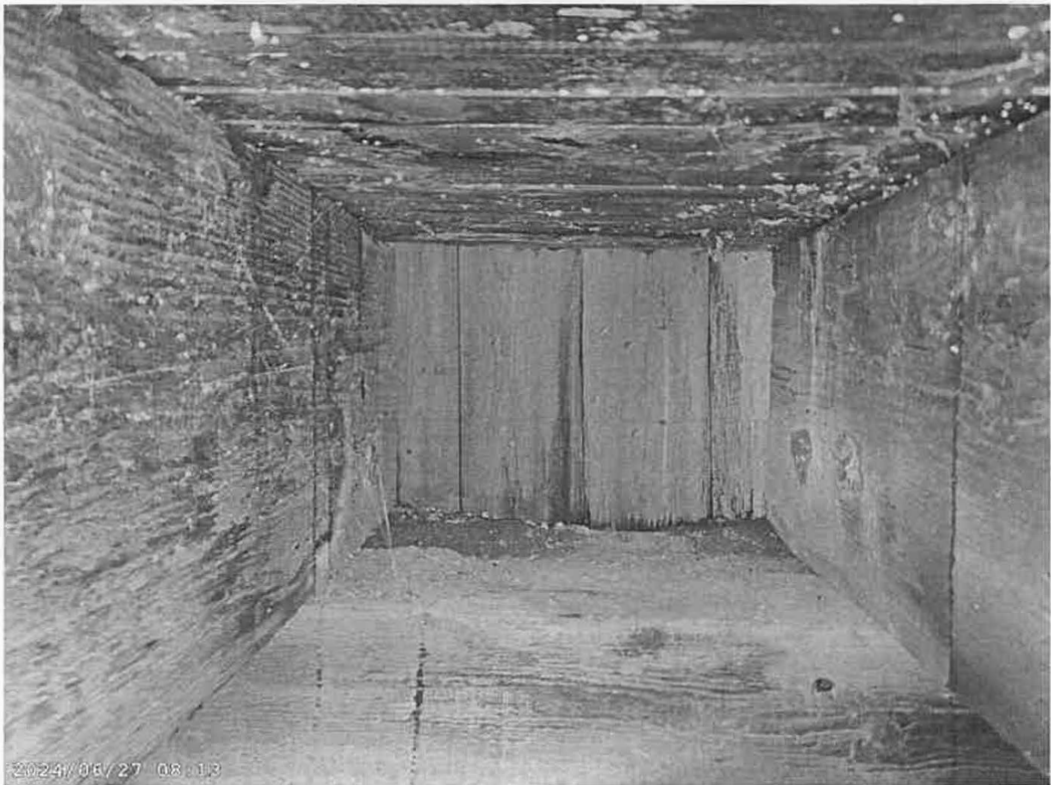
Moderate decay of ballast wall at Northeast corner
