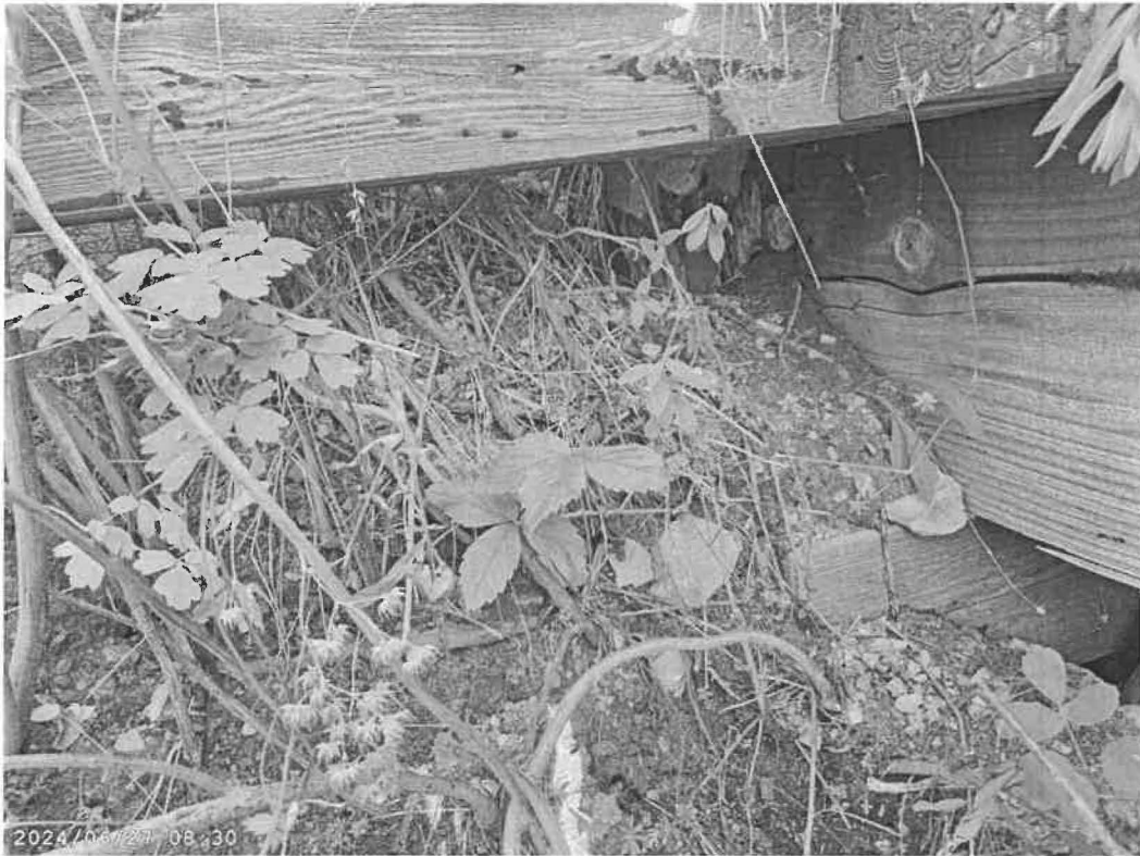
Failed ballast wall corners causing loss of fill onto bearing timber
