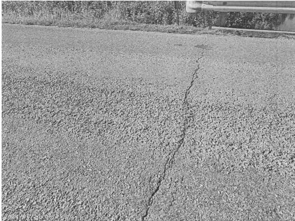
Medium transverse crack at end of deck
