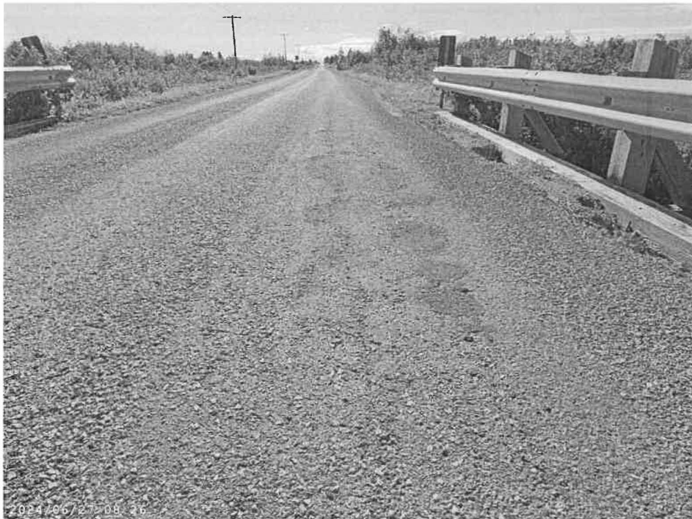
Patching and rutting in wheel path on deck
